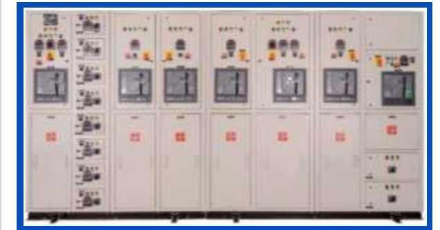
PCC / MCC / VFD Panel
